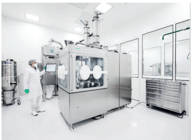
Cleanrooms, a powder laboratory, and state-of-the-art equipment create ideal conditions for trials with capsules and tablets
